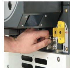
8- Unlock the earthing switch by the key (if available)
