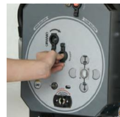
12- Close (ON) the vacuum circuit breaker
