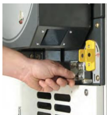
2- Unlock the earthing switch by the key (if available)
