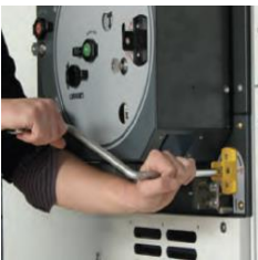
9- Close the earthing switch
