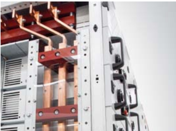
Side bus-bars: placed on the left for the connection of the power supply pliers and the disconnecting switch.
